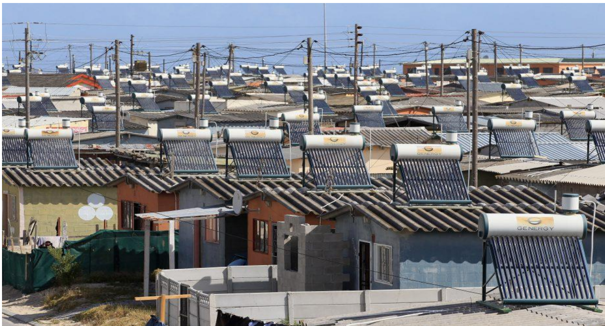
Figure 17: Use of solar energy in South Africa townships
